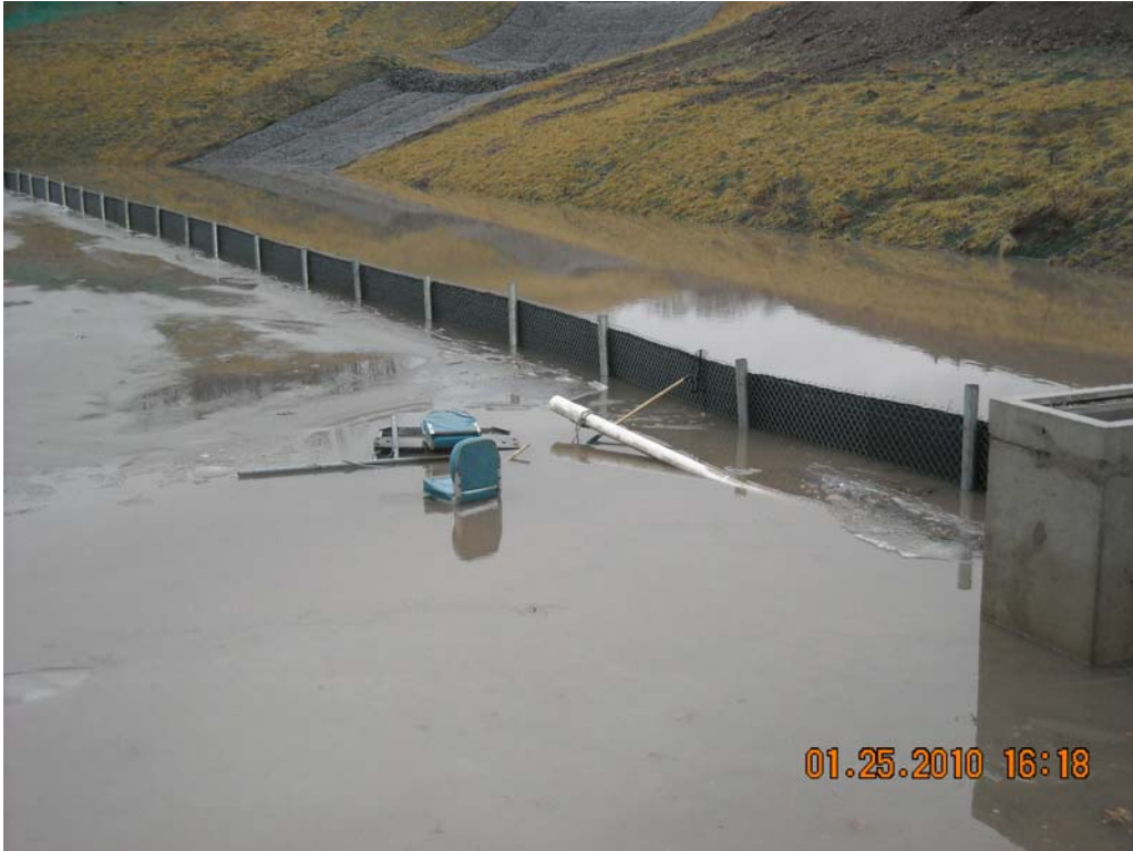
Skimmer arm above water surface 01-25-10
