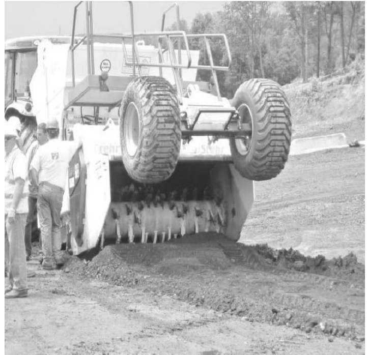
Solidification Equipment—Dust Free Soil Stabilizer
