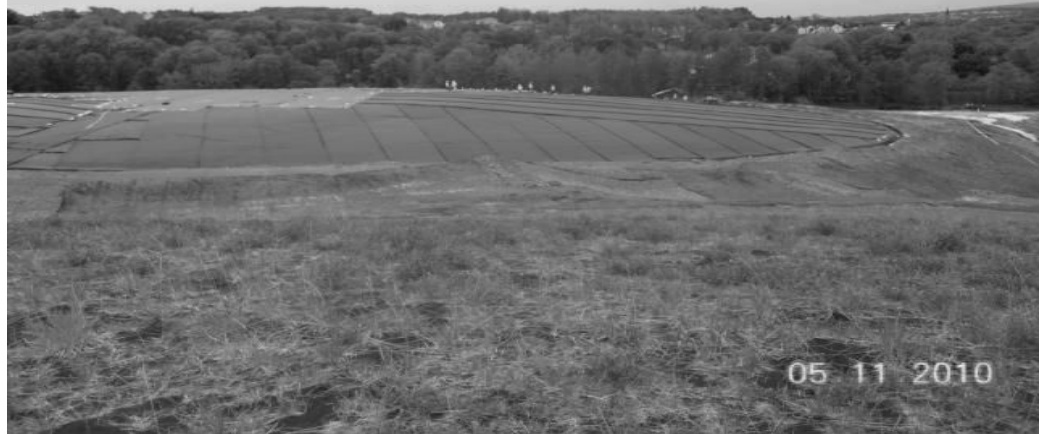
View of geosynthetics installed on the western part of the Containment (Cap) Area — 5/11/10
