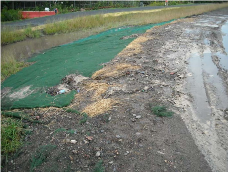
Picture 3: Overflow Area (08-10-09)
