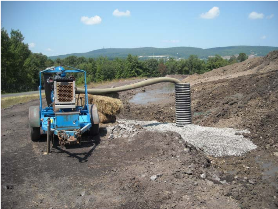
Picture 6: Additional Pump installed (08-15-09)
