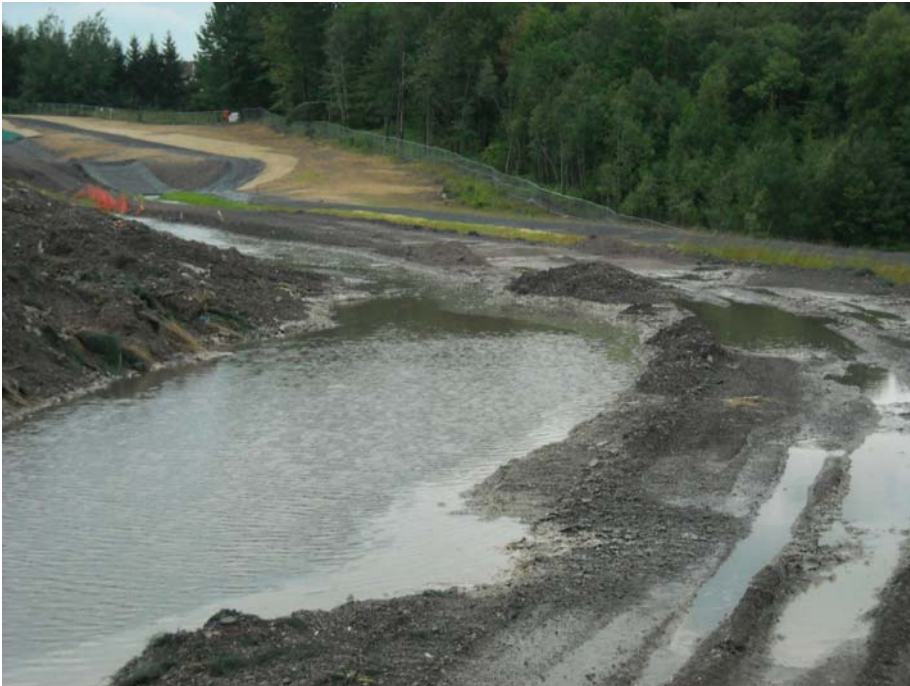
Picture 2: Water overflow along section of CA berm (08-10-09)
